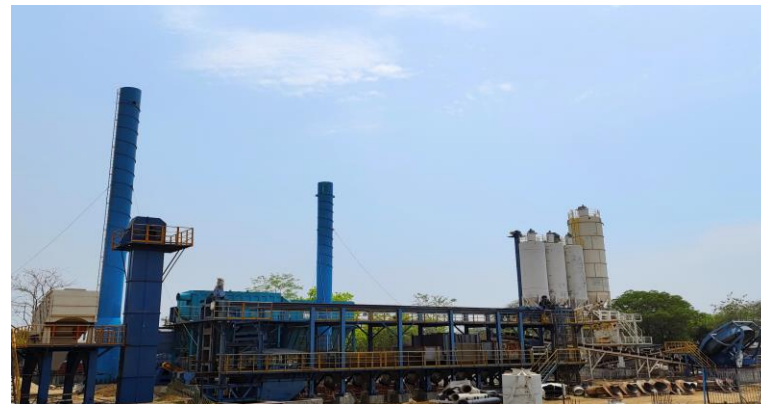
Ash to Sand Facility at NTPC Sipat
